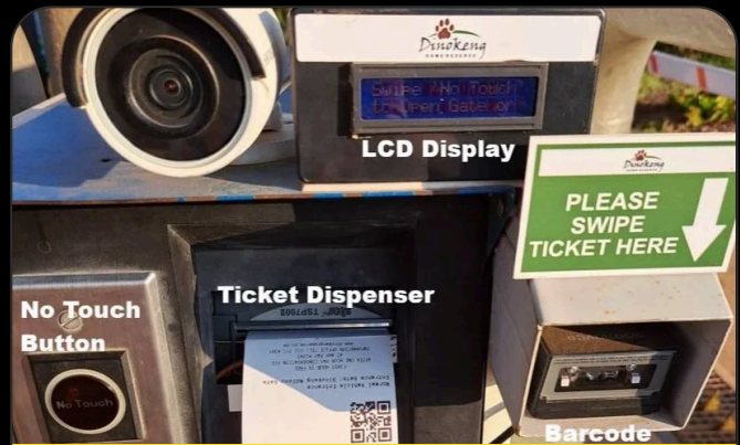
The gate pedestal: 2-line LCD display, No Touch button, ticket dispenser with a QR ticket and barcode scanner.
