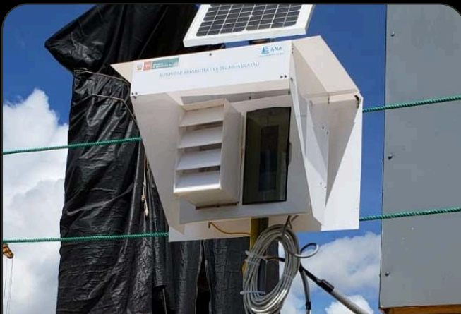
The station on site in Pucallpa: enclosure with the AAA Ucayali and ANA logos and a small solar panel on top.
