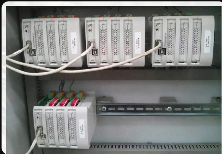
Inside the cabinet at Fortaps: four M-Duino PLCs, each labelled for two lines (1-2, 3-4, 5-6, 7-8), each with its Ethernet cable.
